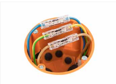
Wiring conductors in a flush-mounted junction box.
