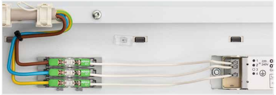
Wiring in the ceiling light.
