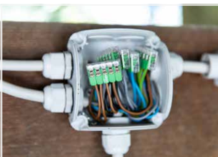
Wiring in the distribution box.
