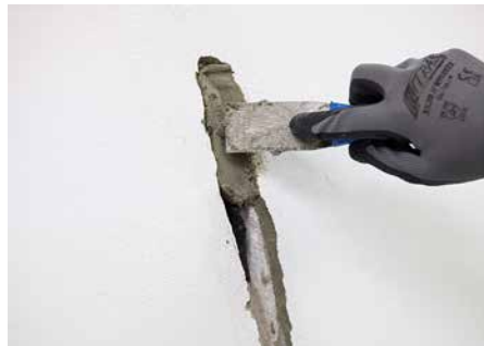
Close the damaged area discreetly.
