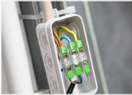
Wiring in the distribution box.
