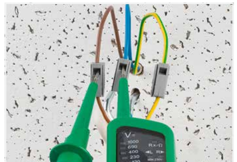
Testing via separate test ports.
